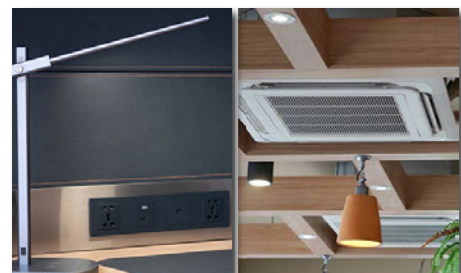
Office outlets Heating system
